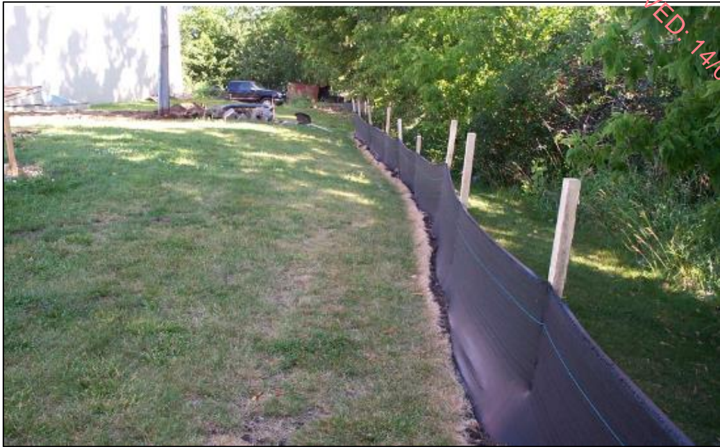
Figure 3.3.1.2.2: Example of silt fence in operation on similar site.
